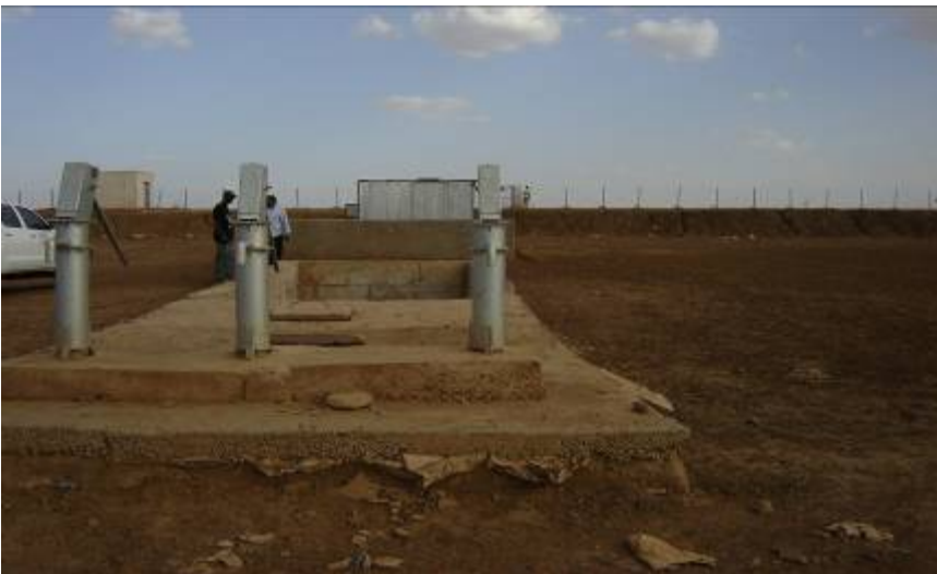
Figure 2. Slow sand filtration system under construction for the hafir at Dar Hashay, Kassala State
