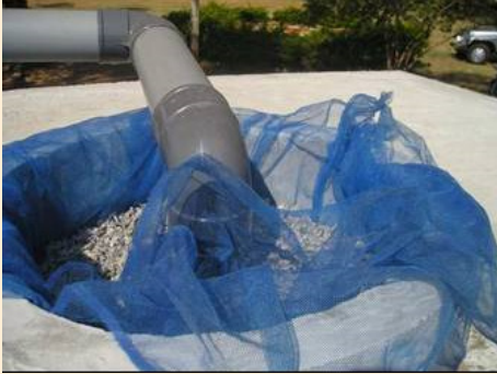
Picture (2.1) Filter at the entrance of tank
