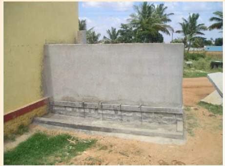
Picture (2.4) Water taps outlet system and cemented area below the tap for letting wastewater disposal
