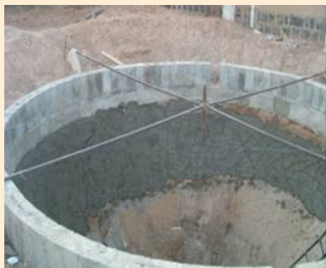
Picture (1.11a) Ferro-cement tank at a girls' school in Sana'a (during construction) (SFD)
