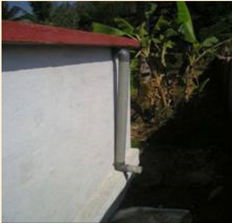
Picture (2.3) Overflow pipe with mesh
